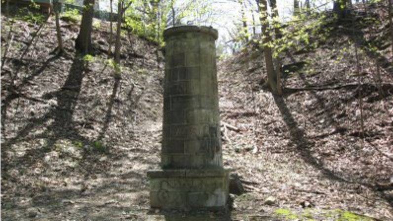
This was the first of three air ventilators, spaced 1 mile apart, we were supposed to pass on our way to the dam. The aqueduct system draws air down from these vents to keep the water flowing toward its destination, while allowing excess air pressure to escape before problems develop. This engineering technique is borrowed from the old Roman aqueducts.
